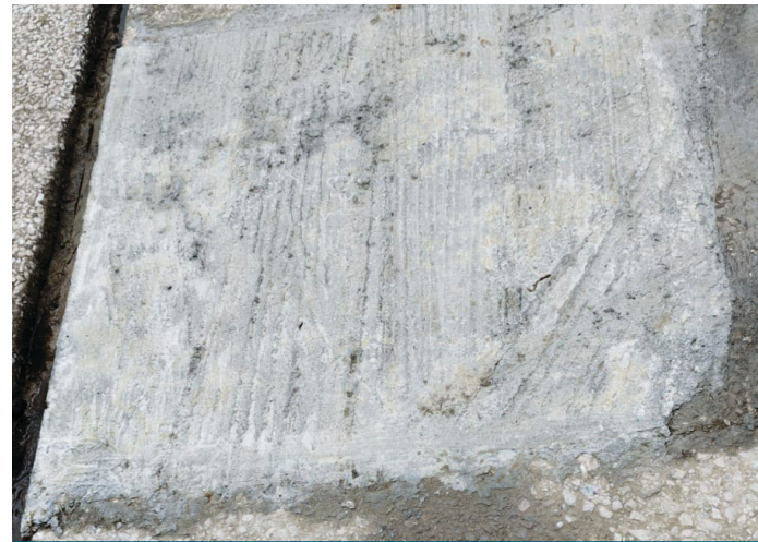
Evidence of Repaired Silage Slab
